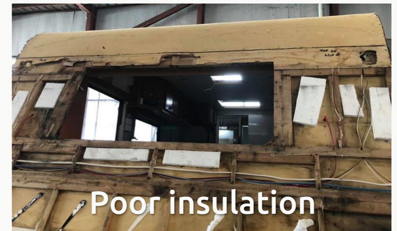
Figure 16 Poor insulation inside Caravan walls (2019) by T. Leigh - Lemon Caravans & RVs in Australia FB group
